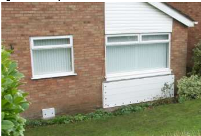
Figure 91: Example of a flood air brick and underfloor flood protection
