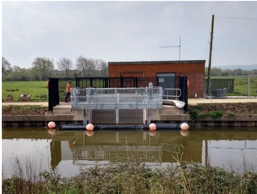
Figure 24 Screen installed in AMP7 under EE_IMP driver near the intake from Bridgwater and Taunton Canal.
