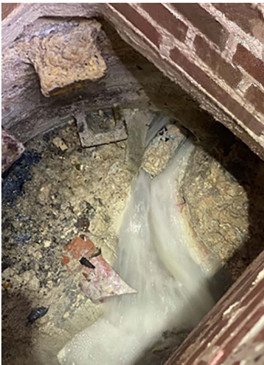
Demonstration of misconnection
