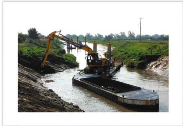
Dredging the River Parrett with floating equipment just upstream of Westonzoyland Pumping Station in 2014 (SRA)
