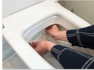
Leaky loo strips
